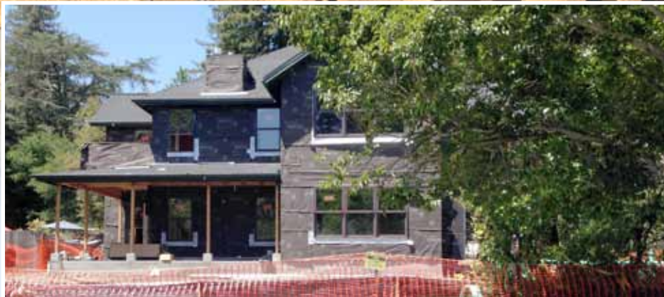
This structure on Bolinas Avenue near the Shaw Guest House will boast two new 3-bedroom single-level homes. By mid-May, the exterior walls were papered in preparation for shingles and all windows were installed.
